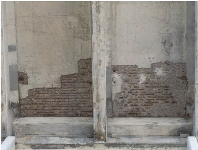
Figure 11. Deck slab bottom contour in the S31-S30 zone next to pier S31, moisture due to seepage at joint after hydrodemolition of damaged concrete [14]
