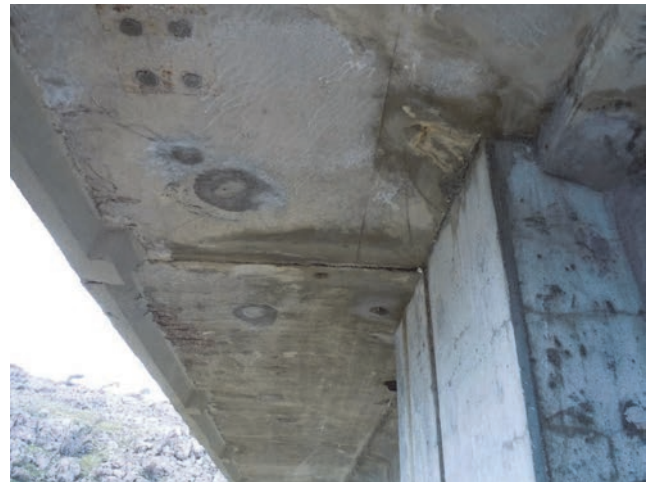
Figure 12. Seepage through joint at pier S30, Crikvenica sidei [14]
