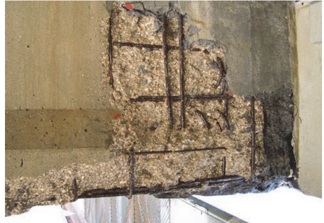
Figure 10. Side of main girder in the S20-S21 zone at pier S21 after removal of poor-quality concrete [14]
