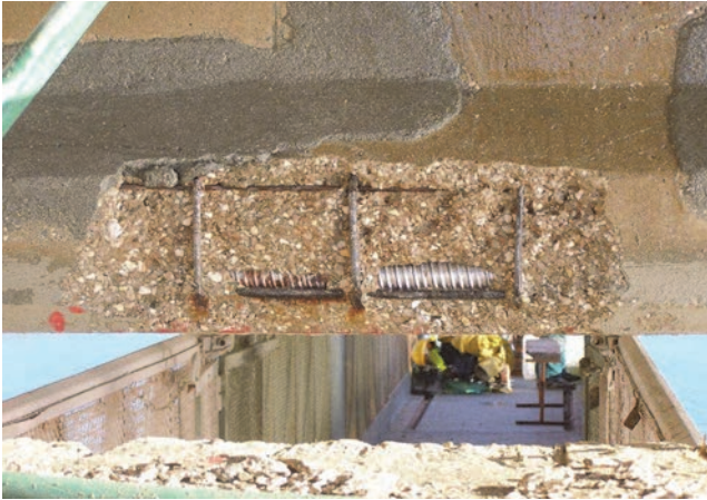
Figure 9. Bottom flange of the main girder in the U4-S20 zone after removal of poor-quality concrete [14]
